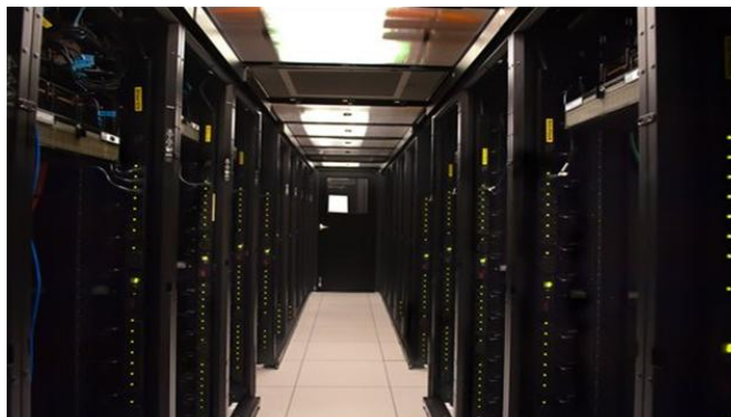
Figure 1. NREL's data center hot aisle containment system. Photo by Dennis Schroeder, NREL/PIX 18781.
